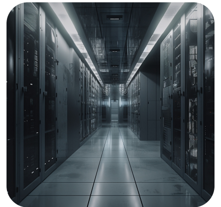
Data Center Cabling
